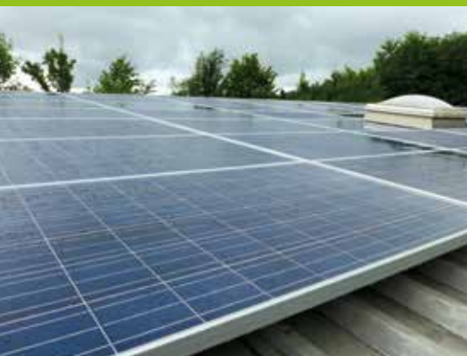
Photovoltaik-Anlage Lindner Hotel & Sporting Club Wiesensee
